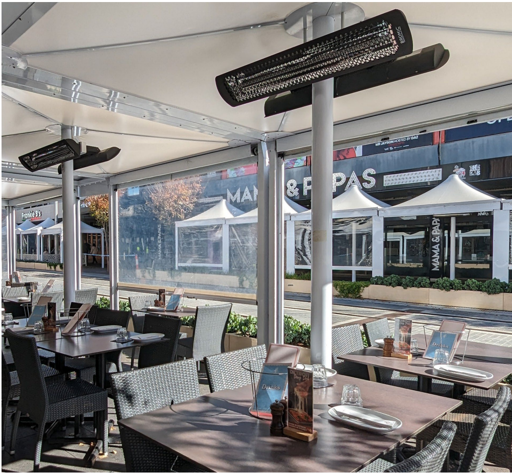
Photo showing heating devices mounted to a structure
