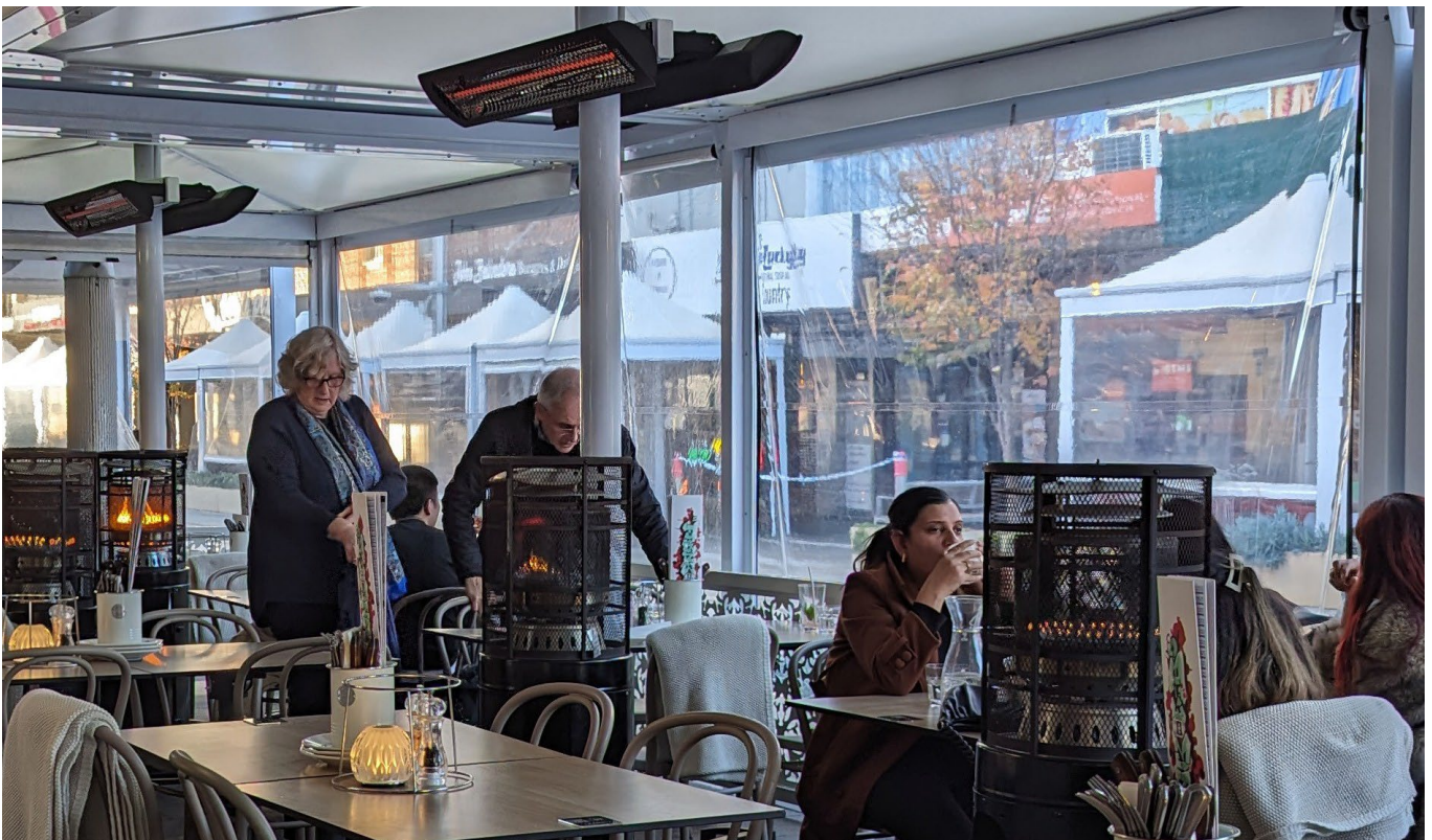
Photo showing standalone heating devices operating to supplement the operation of mounted devices in colder months
